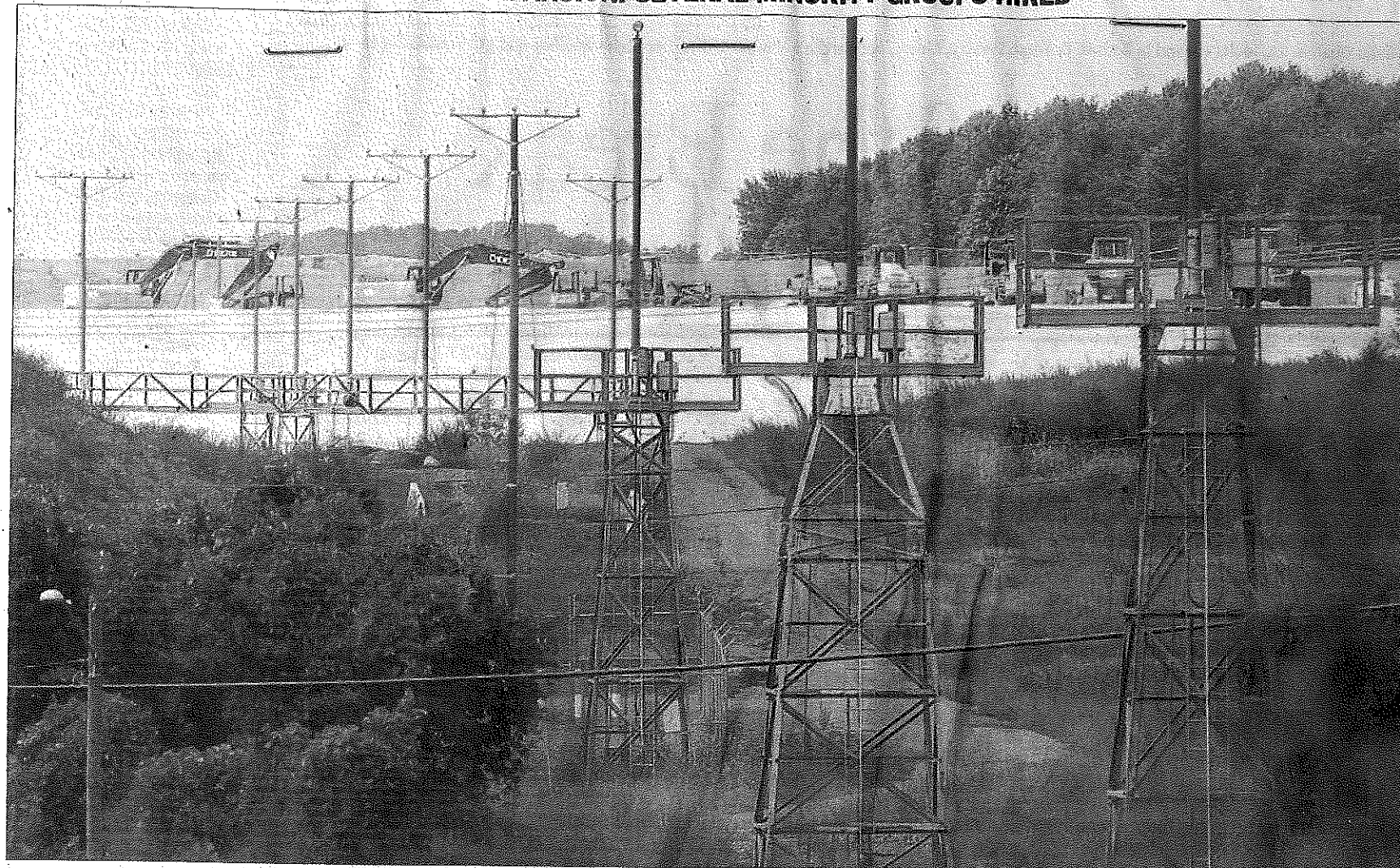
Construction at Smith Reynolds Airport can be seen from New Walkertown Road. A runway is being extended about 400 feet to provide an emergency runover area. JOURNAL PHOTO BY AMANDA MUSCHLITZ
